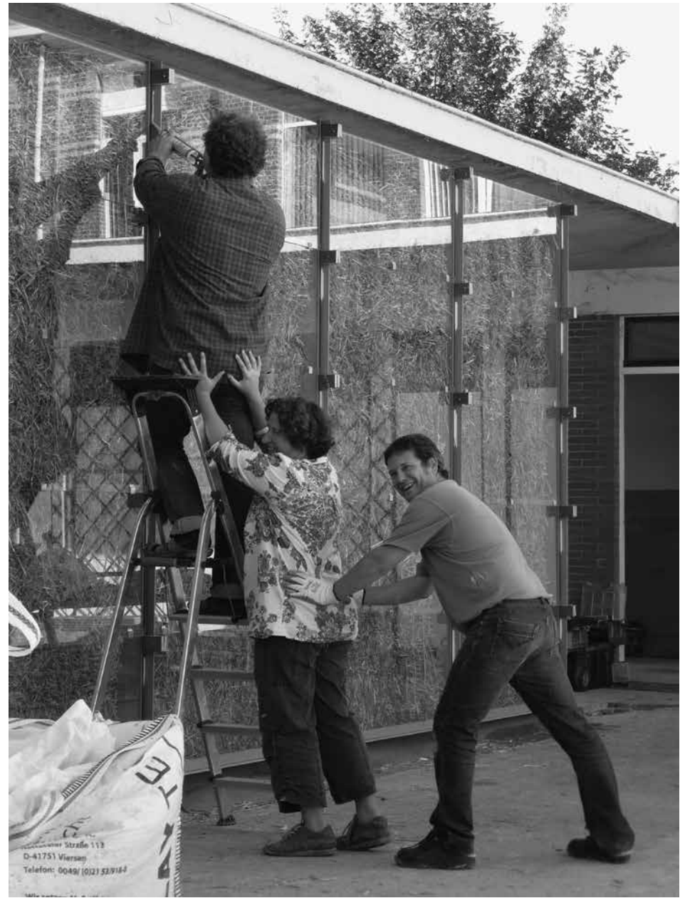
Image: Family and friends constructing the façade Photograph by Wim Goes Architectuur
